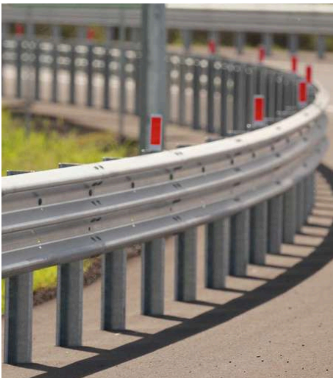
Metal beam Crashbarrier
